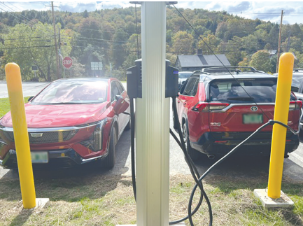
West River Coffee Barn's new dual-port Level 2 EV charger. PHOTO PROVIDED
