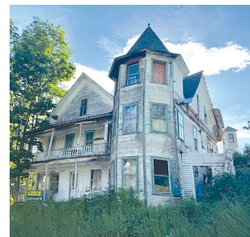
The deteriorating house on the Melendy property in South Londonderry.
