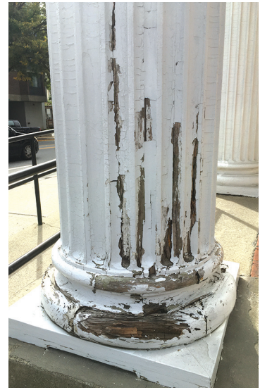
Damage to one of the columns. PHOTO PROVIDED
