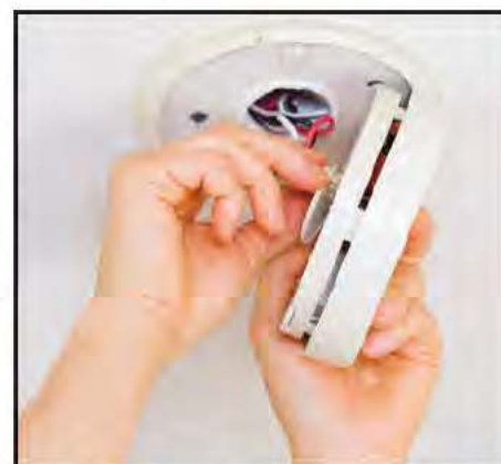
Verify that your smoke detectors are working.
