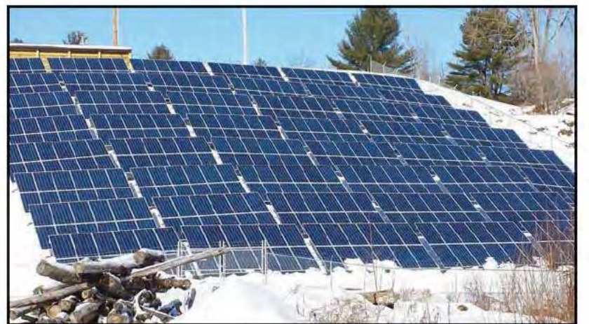
Cavendish town solar array.
