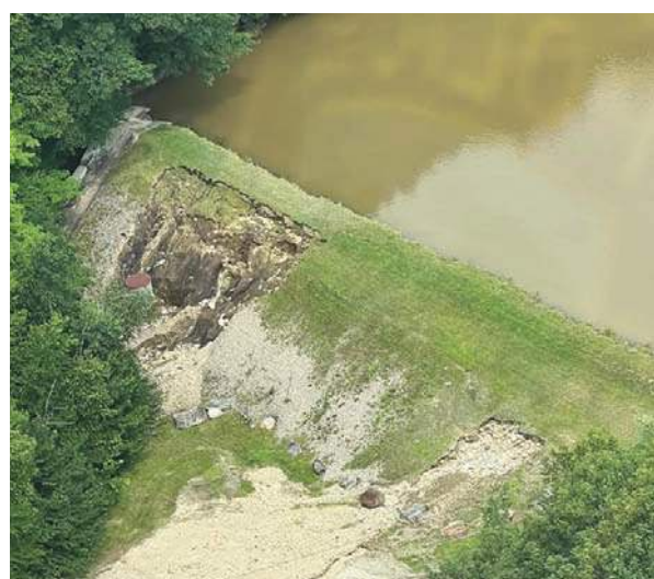
Damage to the Chester Reservoir Dam. PHOTO PROVIDED BY CHESTER POLICE DEPARTMENT
