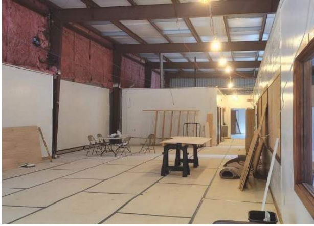
Contractors have removed the interior ceiling and opened many of the walls in the municipal building as of June 16. PHOTO PROVIDED
