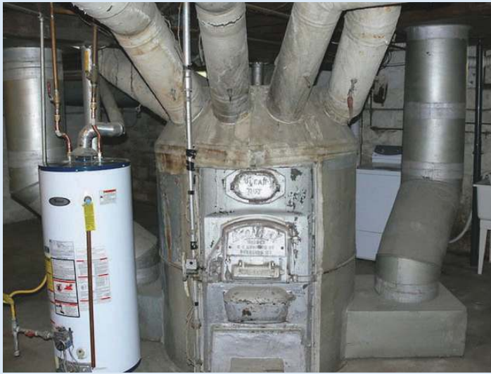
Coal furnace showing octopus arms.
