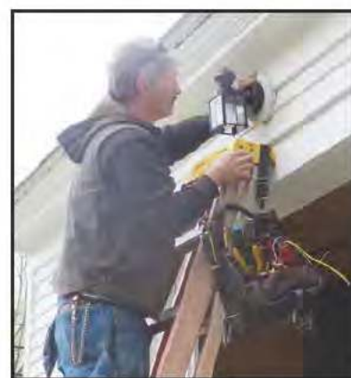
Steve Mancuso of Chester Electric installs an outside light on the Hearse House.
